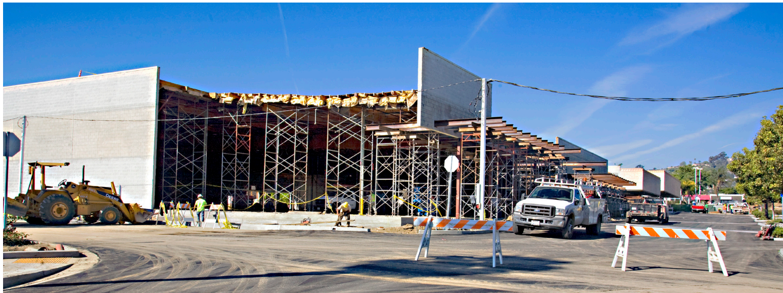
Upgrade and Renovation Pacific View Mall. New Trader Joes, Bevmo, and more.
